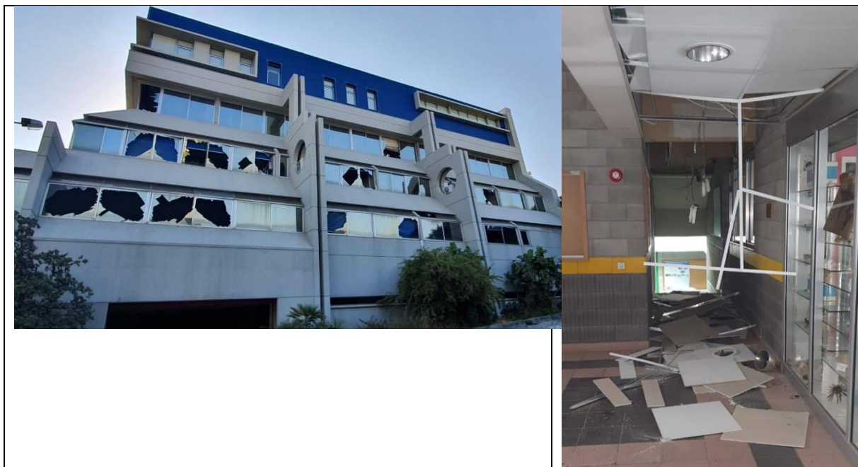
Figure 9 : Illustration of damages generated by the blast (6 th August 2020) at USJ.
